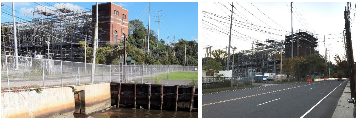
CSHH #14A, powerhouse drain outfall (l) adjacent to the lot that was the site of the old brick powerhouse building; demolition of brick structure (r) on east side of the road (photos by Carol DiPaolo, 9/2/21, and Michelle Lapinel McAllister, 10/22/22, respectively)
