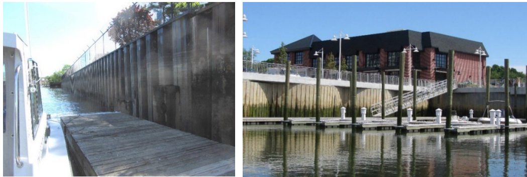
New bulkhead below STP on south side of Glen Cove Creek (l) and Glen Cove Brewery near completion on north side of Glen Cove Creek (r) (photos by Carol DiPaolo, 5/18/22)
